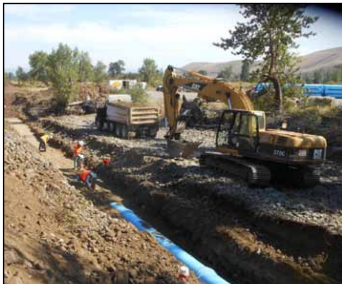
Construction of a new irrigation pipeline near Manastash Creek, which will help ensure water for both salmon and farmers.
