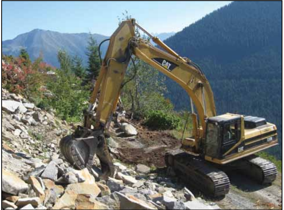
A large excavator, high above I-90 exit 47, begins to place a mountain bike trail over a forest road. Granite Mountain is in the background.
