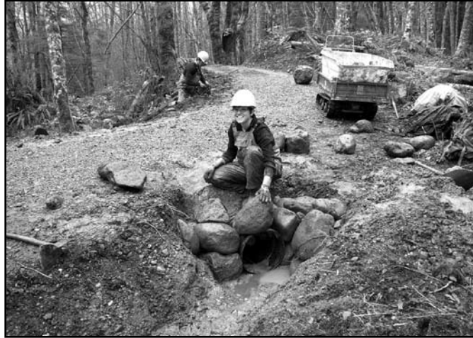
Greenway field crew members Addie Candib (foreground) and Cameron Shaughnessy (background) put the finishing touches on a new drainage culvert on the W. Tiger #3 Trail.
