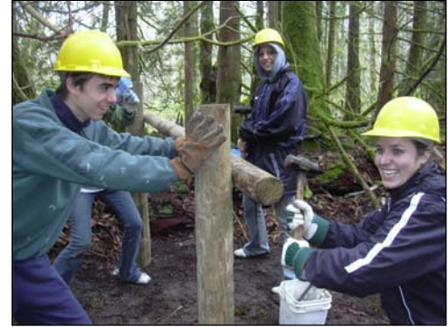
Volunteers installed new signs, gates and bridges to improve Tiger Mountain trails.
